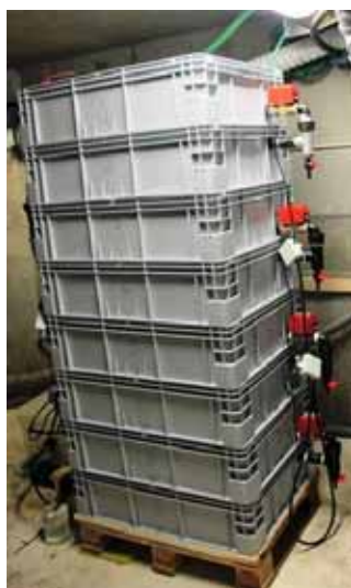
Figure: Greywater treatment plant tower
